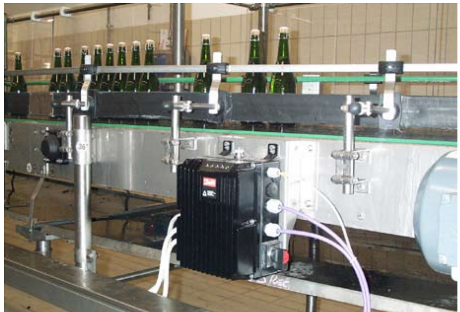
IP66 VLT® decentral FCD 300 drives mounted near by the motor
