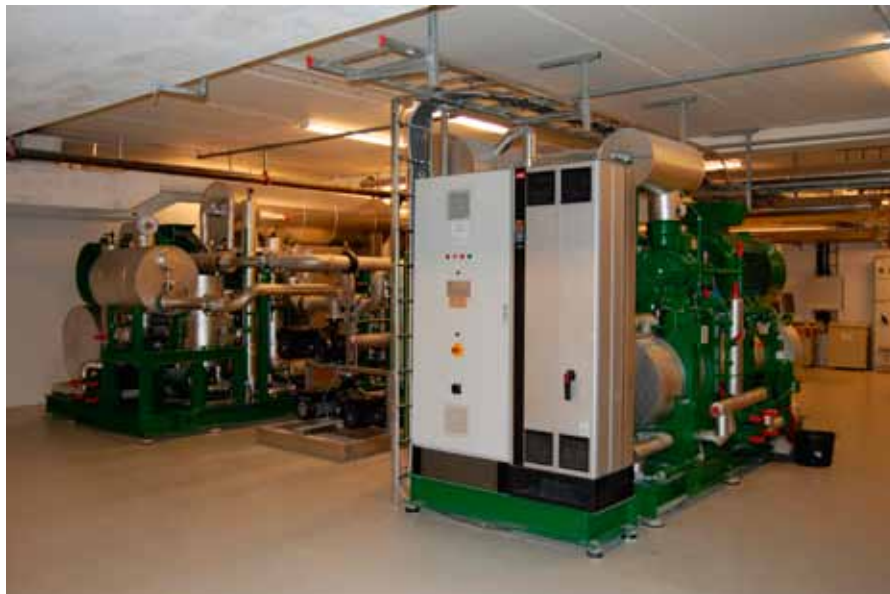
Two 355 kW VLT® HVAC Drives FC 102 IP 54 frequency converters control the screw compressors which enable the two GEA Greenco heat pumps with a combined performance of 2,400 kW to adjust the heat capacity continuously from low to full performance, with the same efficiency.
