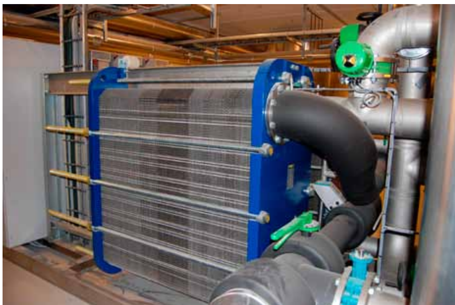
The cooled water from the heat exchanger is circulated in the building to cool rooms to the desired temperature. No active refrigeration is required.
