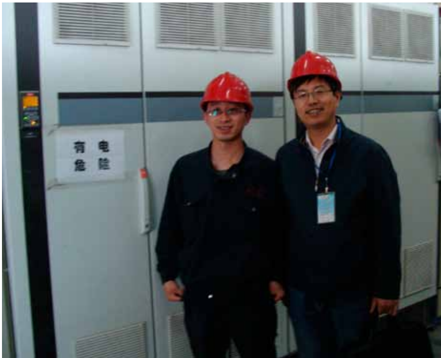
Mr. Guan Mingqiang, electricity engineer at Erdos Chemical Group and Mr. Zhao Wanjun from Danfoss in front of the installed VLT® drives.
