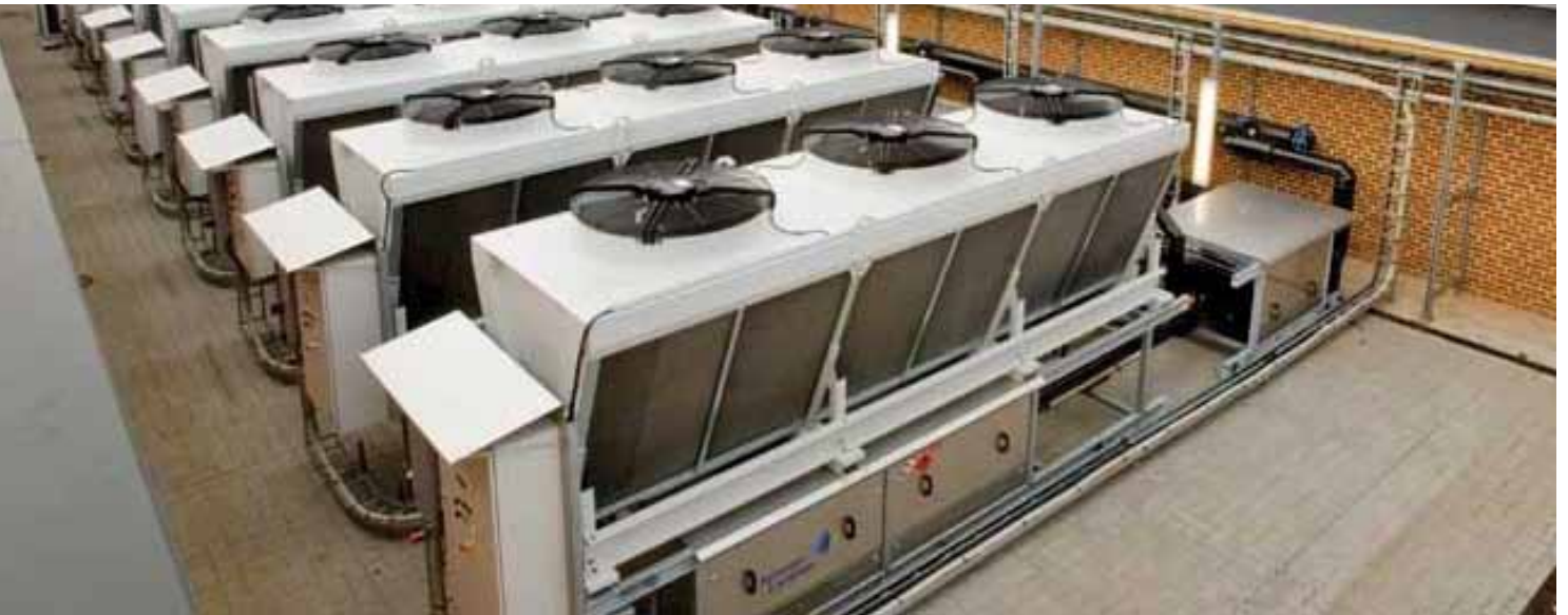
Environmental chillers in roof-top installation at Aarhus University Hospital. On each chiller are installed a VLT® HVAC Drive FC 102, 90 kW, IP55 enclosure and a VLT® HVAC Drive FC 102, 5,5 kW, IP55.
