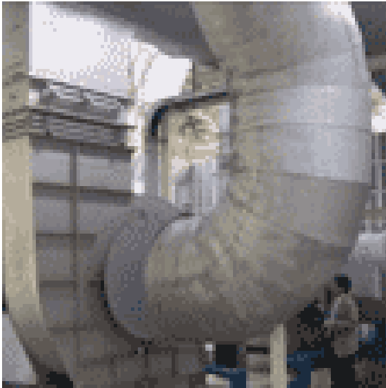
The ID fans in the Korean incinerator plant
