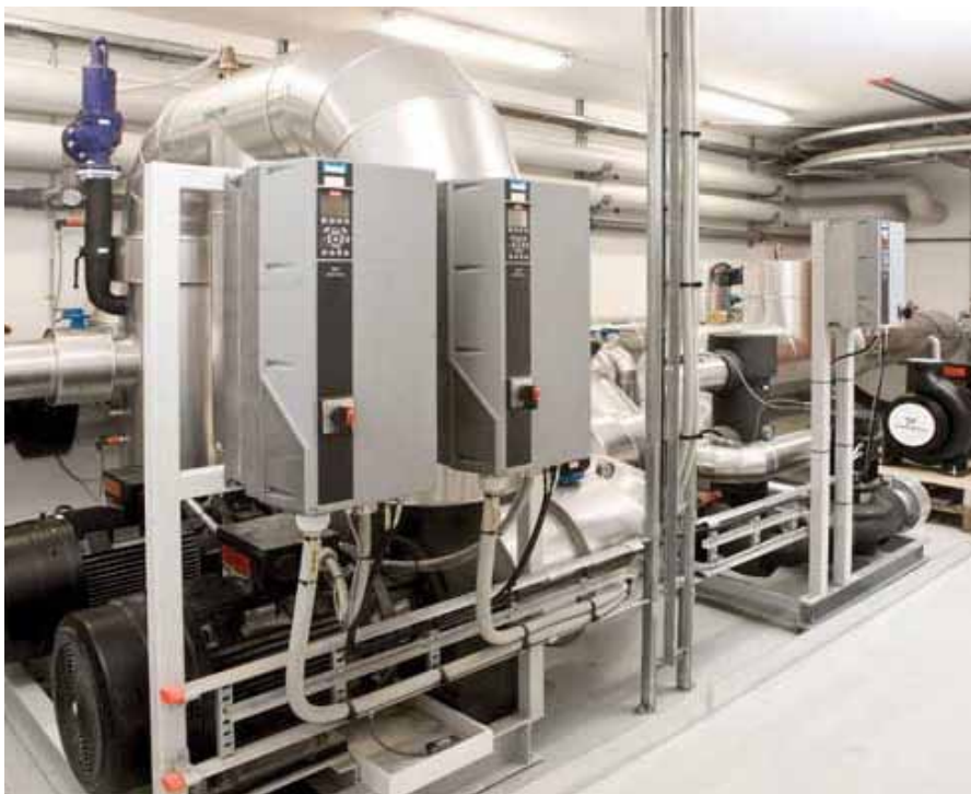
VLT® HVAC Drive FC 102, 37 kW, IP55 enclosure installed on each heat pump.
