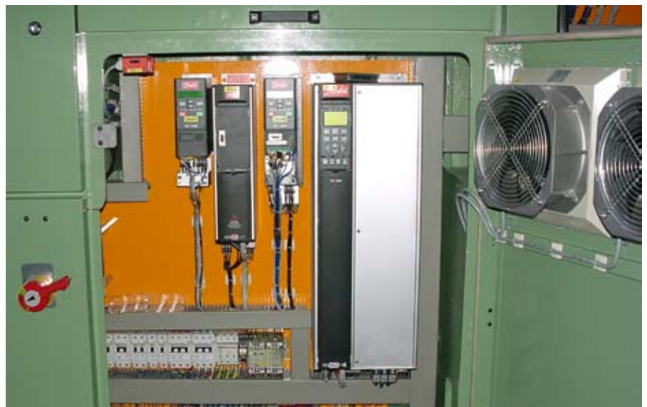
The compact VLT® drives mounted in a air conditioned cabinet
