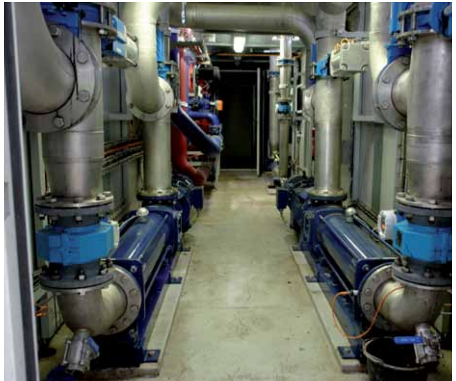
Seepex progressive cavity pumps powered by Danfoss VLT drives.
