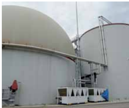
The manure digestion tanks (6,000 cubic metres per tank) hold sufficient biomass for 10 megawatt generation capacity.
